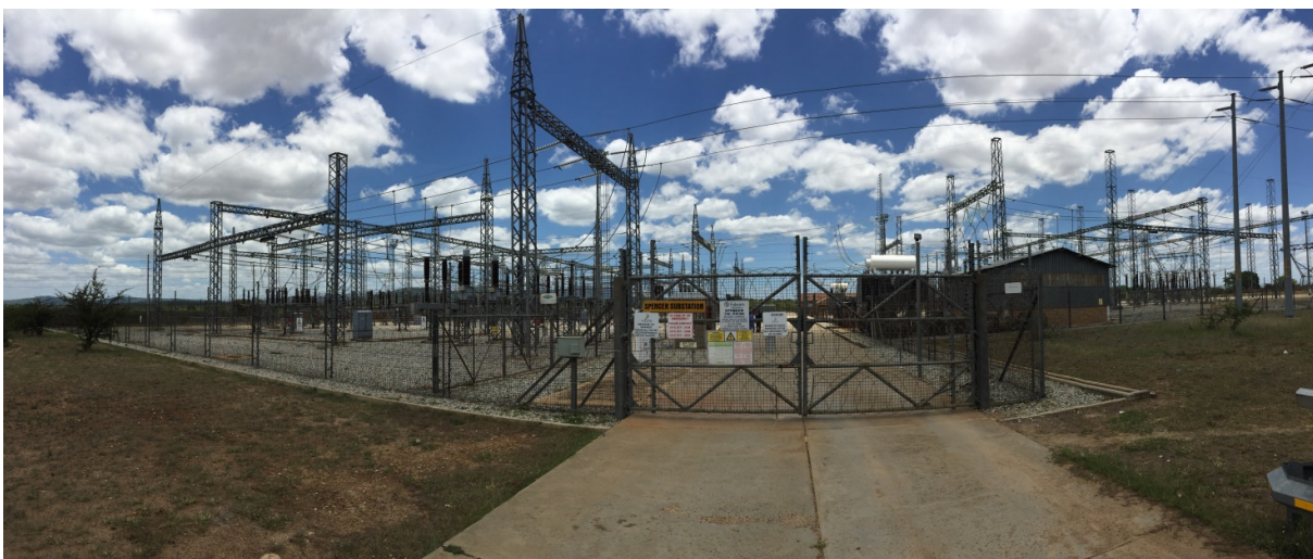
Figure 10: Photograph of the Spencer substation.
